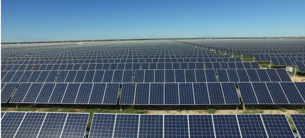
Utility-scale solar project. Source: Xcel Energy.
